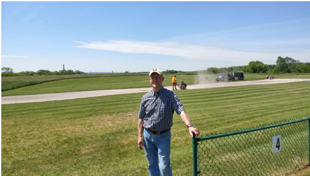
Brian Harrington in front of runway as work is being carried out.
